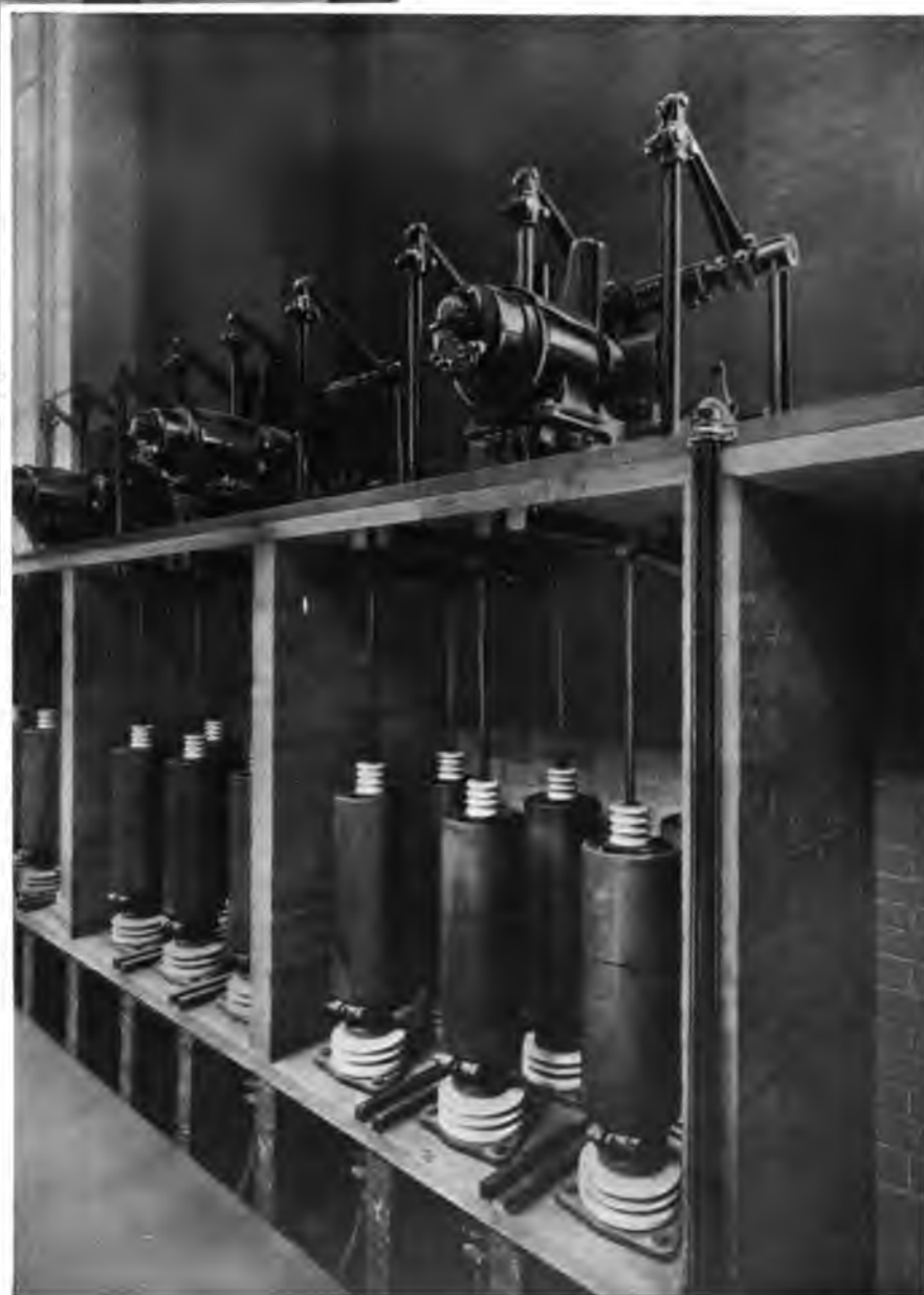
OIL SWITCHES — MAIN POWER STATION
